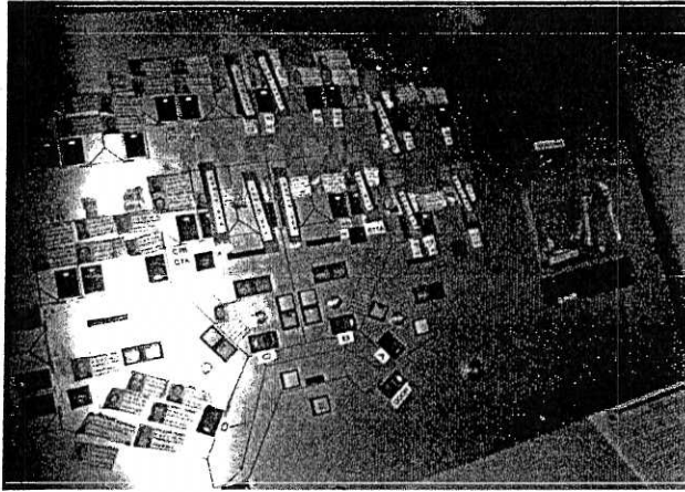
Housing Unit Door Control Panel
